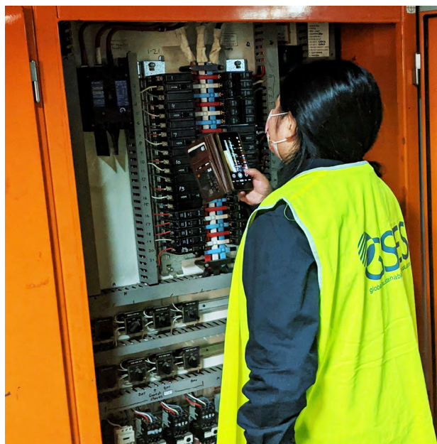
Figure 19: A qualified engineering professional checking the main switchboard
