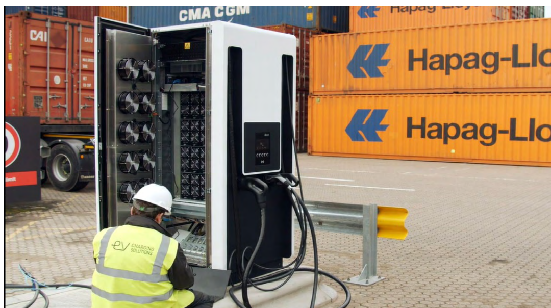
Figure 24: An electrician conducting maintenance for an EV charging station
