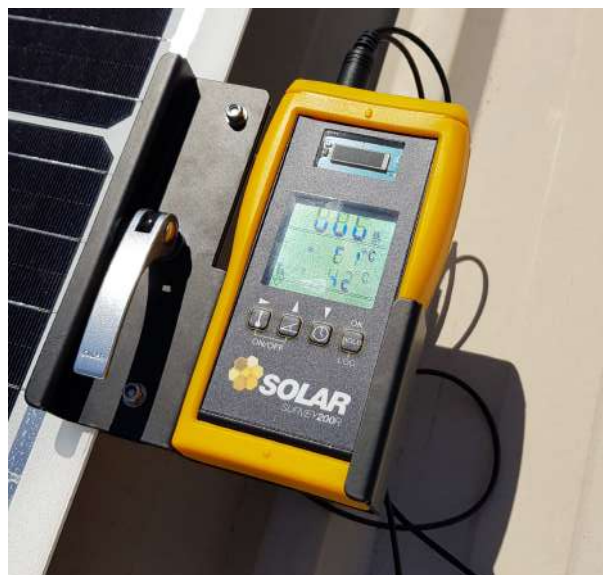
Figure 4: IV Curve sweep in progress
