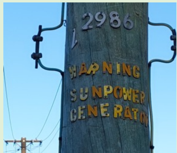
Warning sign on Transformer Pole-Installed 1997 still there in 2022
