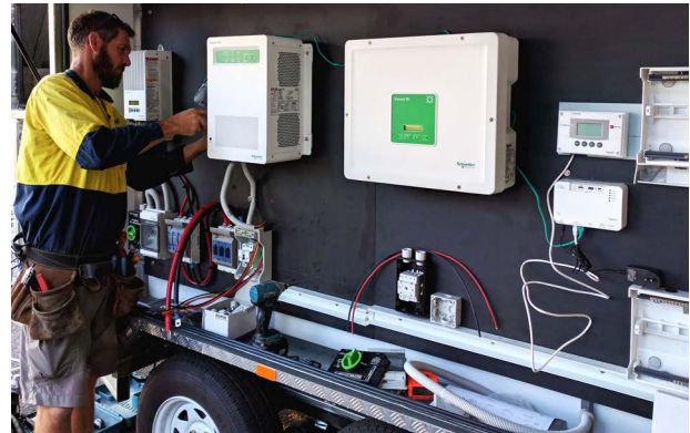
Figure 1 - Installers and designers of grid-connected battery systems undergo nationally recognised training as part of the CEC Accreditation program
