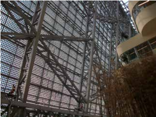
Figure 2: Photovoltaic solar curtain wall at Suntech HQ. (Source: Suntech)
