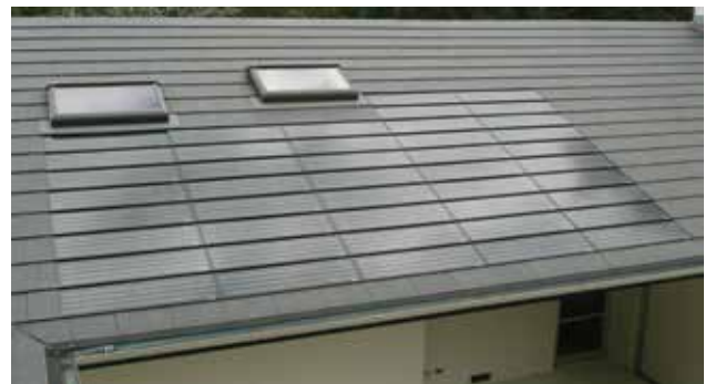
Figure 1: Solar tiles subtly integrated into a roof. (Courtesy: Nu-Lok Roofing Systems.)
