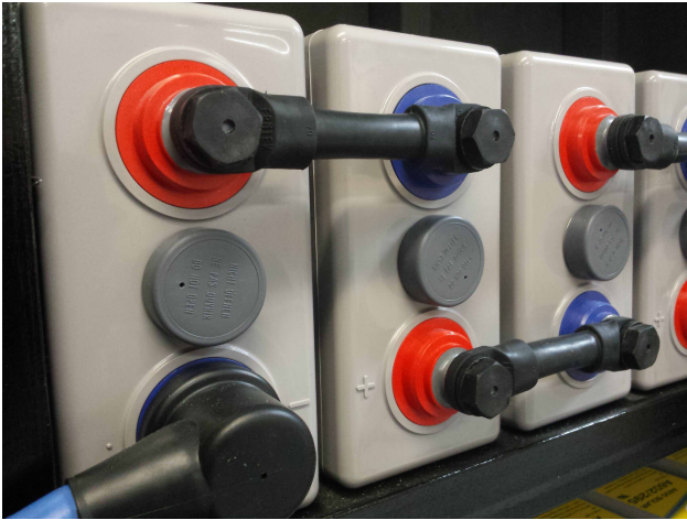
Figure 1: Sealed Lead Acid Batteries in the GSES training centre.
