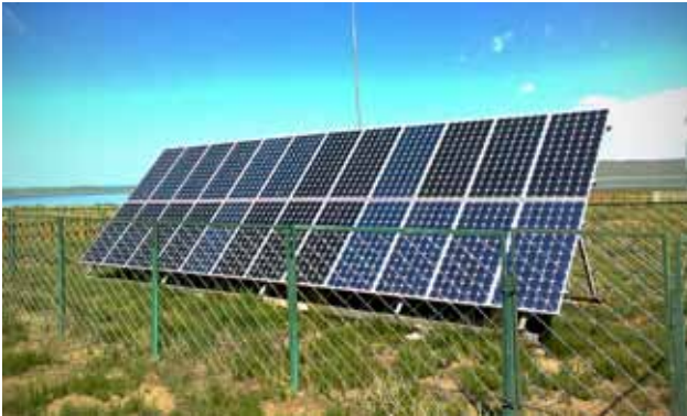
Solar panel installation at an information center adjacent to Ögii Lake (Chinnee, Creative Commons Attribution-Share Alike 3.0 Unported, https://en.wikipedia.org/wiki/File:Solar_panels_in_Ogiinuur.jpg )
